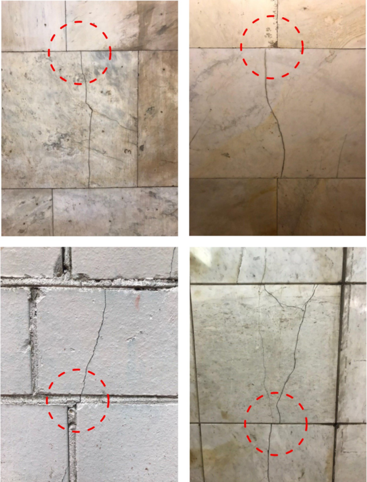
Figure 2. Examples of cracks in building tiles.
