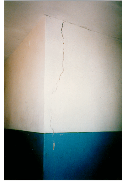
Figure 5. Crack in plaster in separating brick wall on ground floor of two store brick building. Foto is taken in village Manichskiy. The intensity in this village is assessed to be 6.
